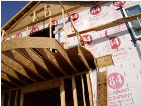
Initial point of impact. Balcony was partially damaged. Also noticeable are the burn marks on the house wrap. (Overall view of the structure)
