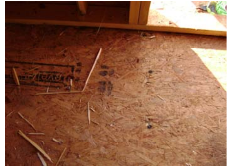
Notice the charring around the nails of the floor joists. The nails were heated to the point that the surrounding area would have been fuel if the floor joists were not treated. (Second level flooring)
