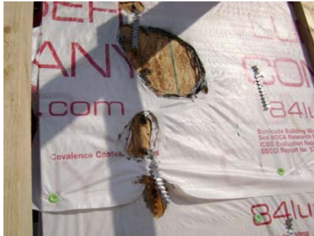
Lightning strike came and hit sheathing. Burn damage noticeable to house wrap. (Close up view)
